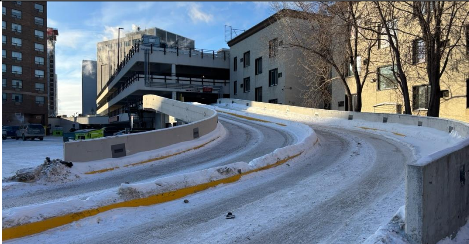
Image Description: A steep ramp leading into The Rice Centre parkade. Snow is on the ground.
